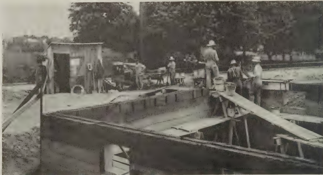
A DOUBLE-WALLED RESIDENCE IN COURSE OF CONSTRUCTION MOLDING MACHINE SHOWN IN POSITION ON FAR WALL. NOTE NECESSARY EQUIPMENT, CONSISTING OF WHEELBARROWS, PAILS, SHOVELS, MIXER AND WATER BARREL. ANGLE IRON GUIDE CAN BE SEEN AT CORNER OF WALL
